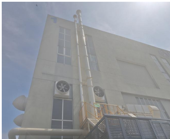
DA001 排气筒/DA002 排气筒
